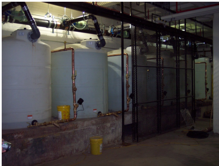
Figure 2-2. Typical plastic cisterns.
