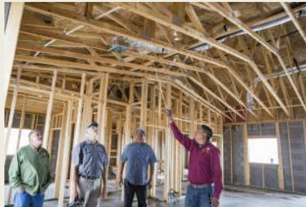
GRIC Staff leading a site tour of homes under construction as part of the technical assistance provided by EPA's MVD initiative. Photo: Gila River Indian News/Christopher Lomahquahu
