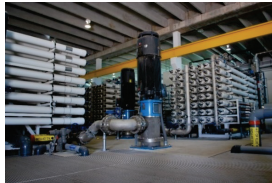
Figure A.6-2 B. RO modules (Photo credit: City of Wichita Falls)
