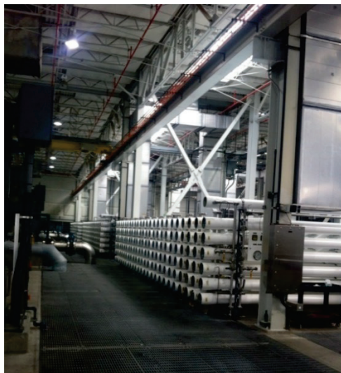
Figure 6-3. RO system at OCGWR
