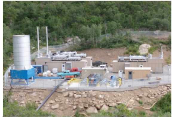
Elk Creek CMM Electric Power Project
