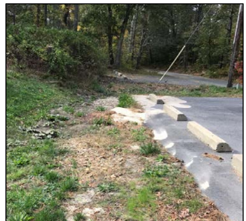
Sediment beyond BMP at Tennis Courts
