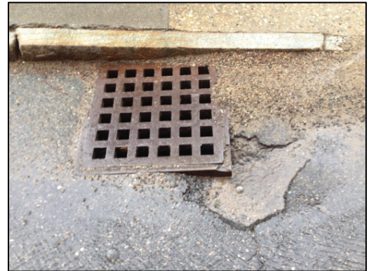
Sediment Buildup at Catch Basin
