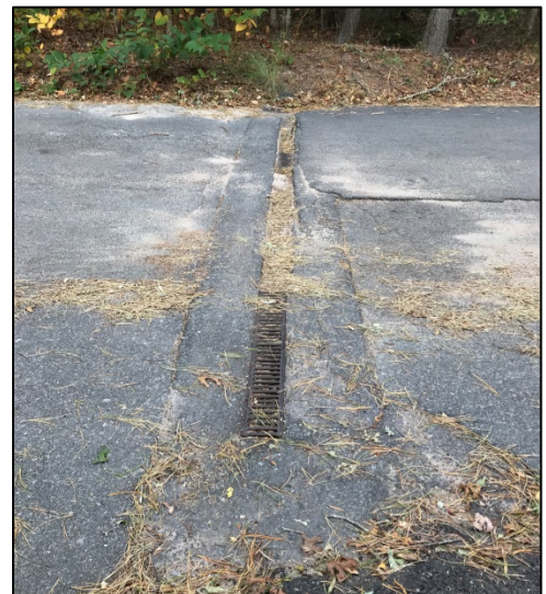
Trench Drain Across Lake Street
