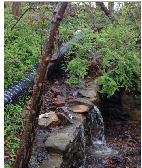
Leaking CMP pipe at Causeway Rd
