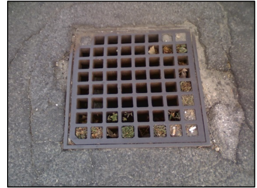
Clogged Catch Basin 195 – Union St
