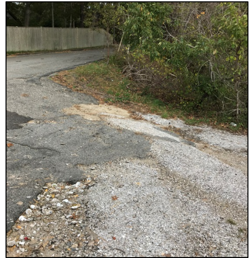
Washout at Landing – East Side
