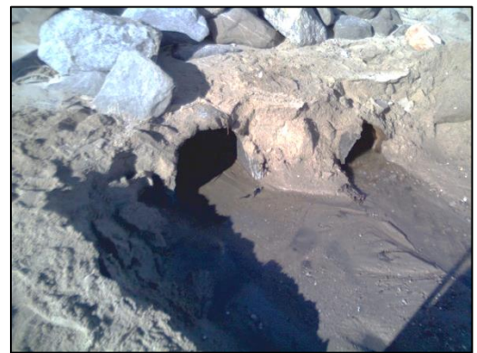
Two Outfalls Uncovered on Beach
