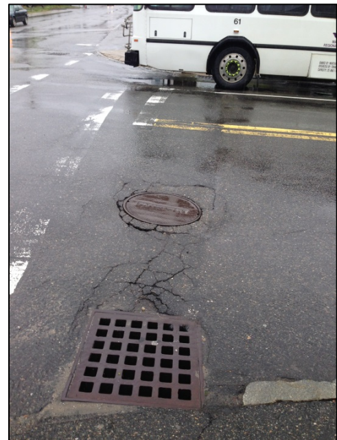
Undermined Structures at Intersection
