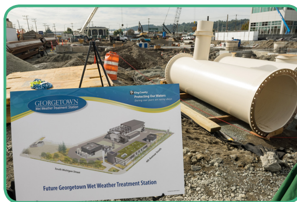
Construction underway at the WIFIA funded Georgetown Wet Weather Treatment Station in King County, Washington
