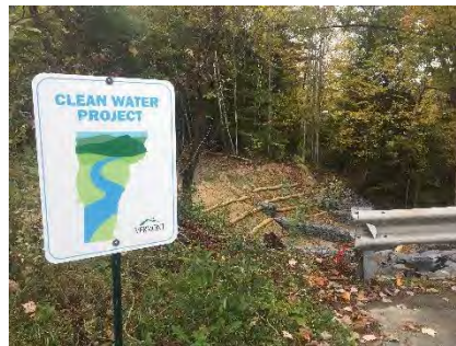
Gully erosion remediation at Pouliot Avenue, Barre Town , completed by Friends of the Winooski River
