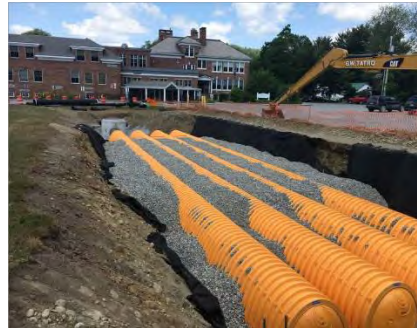
Construction of stormwater treatment practice at Cambridge Elementary , completed by Cambridge Town
