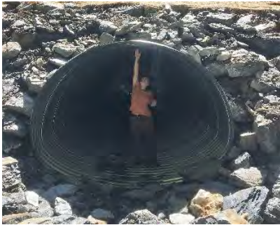
Culvert replacement on Cotton Brook Road , completed by Department of Forests, Parks and Recreation
