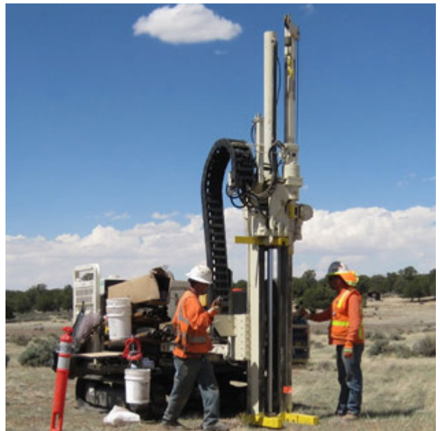
Geoprobe taking soil samples 10 feet below the surface at the Mariano Lake Mine.
