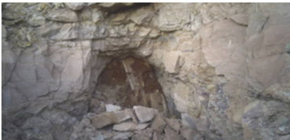
The Navajo Abandoned Mine Lands Reclamation Program closed portals like the one shown here at the Charles Keith mine.
