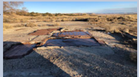
Before and after photos of hazards mitigation work by iina'ba' at Black Jack #1 Mine completed in 2018.
