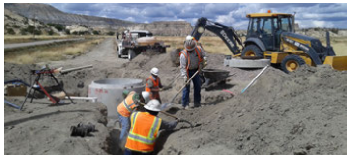
Workers from Navajo Engineering and Construction Authority construct this IHS funded water line extension to provide first service of safe drinking water to 26 homes in Cottonwood.
