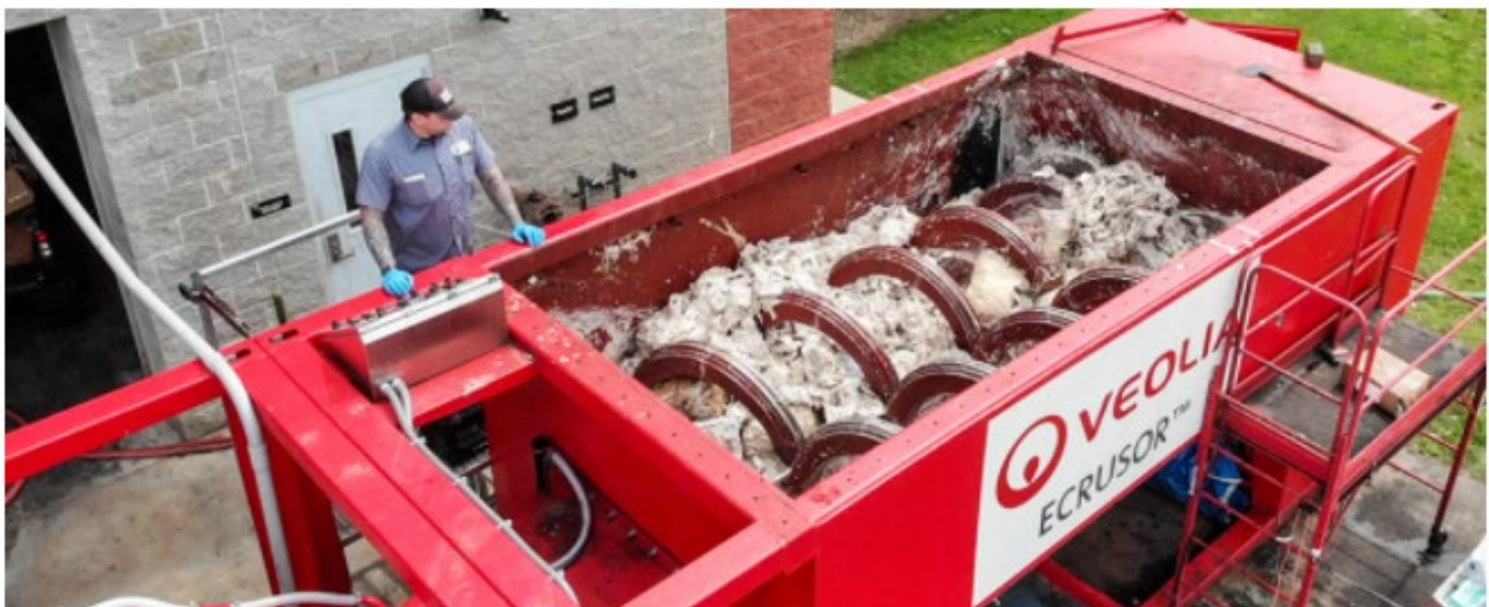
Photo Credit: Thomas Darby, Water Pollution Control, Hermitage, PA
