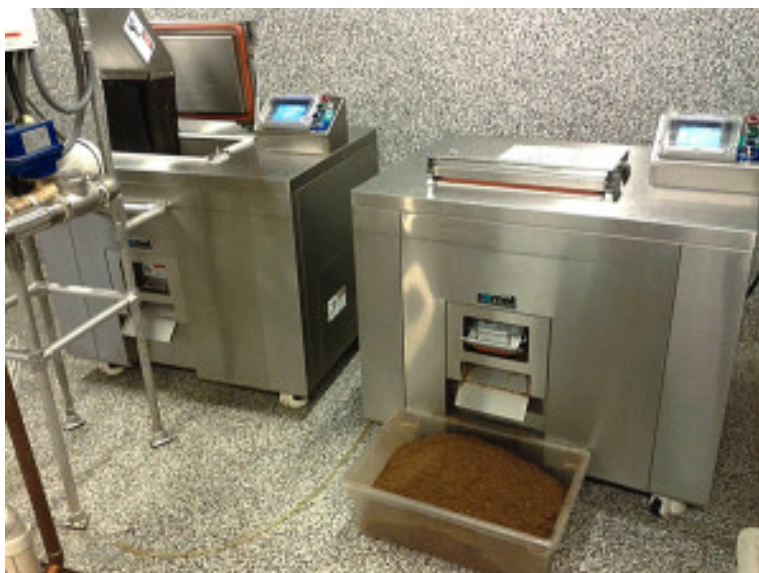
FIGURE 8. SOMAT DEHYDRATORS, ST. CLOUD HOSPITAL, MINNESOTA
