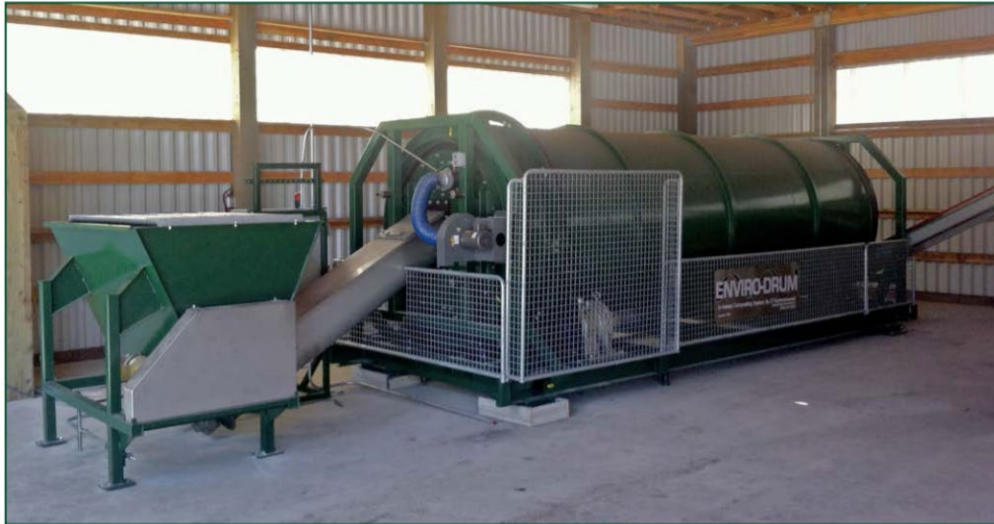
FIGURE 10. DT-ENVIRONMENTAL ENVIRODRUM AEROBIC IN-VESSEL UNIT
