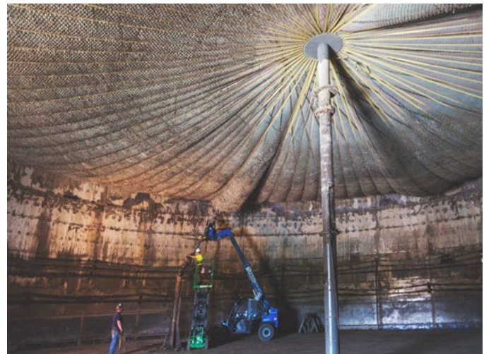
Inside an anaerobic digester at Dane County’s Vienna facility. Photo Credit: Brightmark
