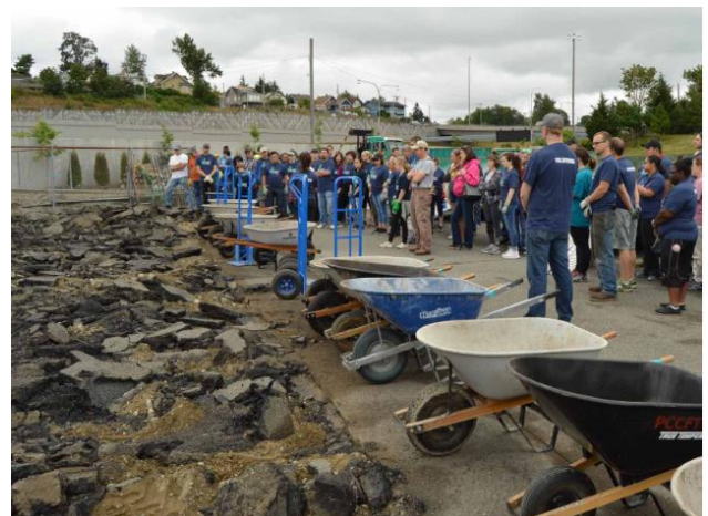
VOLUNTEERS GET READY TO HAUL AWAY PIECES OF ASPHALT DURING A DEPAVING EVENT AT A SCHOOL IN TACOMA. (DEPAVE PUGET SOUND/ CARAVANLAB)
