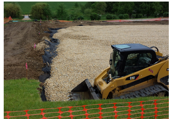
The gravel layers installed before the permeable pavers help to create space to filter and store parking lot runoff.
