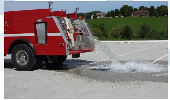
A demonstration of the permeable pavers capturing water.
