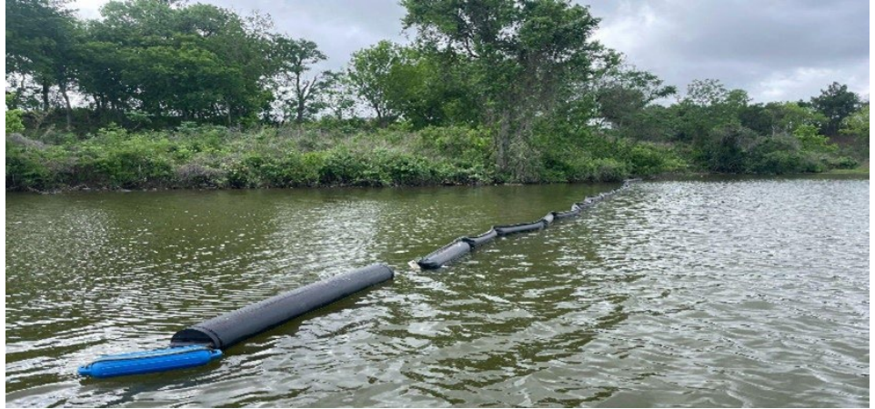
Litter boom system installed in the Houston-Galveston watershed.
