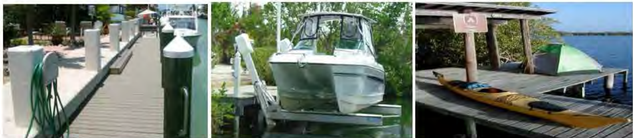
Figure 11. Pile-supported Structures. Example of a marginal dock on the left, boatlift with I-beam in the middle, and a chickee on the right. (The left and middle photos were provided by the Florida Marine Contractors Association and right photo from www.cnn.com ).
