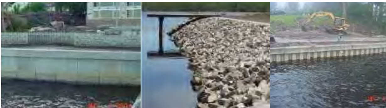
Figure 9. Example images of shoreline armoring and stabilization. The left image is a concrete slab seawall, the middle is a riprap shoreline, and the right is a vinyl seawall. (Images provided by the Florida Marine Contractors Association in 2014).
